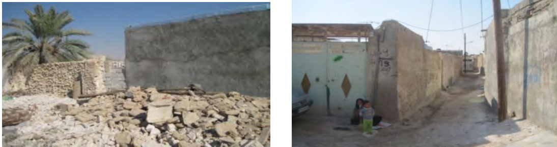
Fig. 3 and 4: Physical erosion in deteriorated areas of Borazjan
